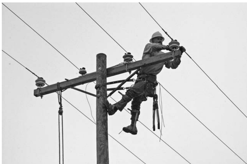
CAMERON, LA, NOV. 2005 A lineman repairs damage from Hurricane Rita. MARVIN NAUMAN/FEMA photo
